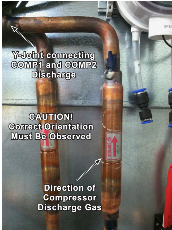
Figure 24: Discharge Line Check Valves on Large Cabinet (7.5T) Heat Pump (DPH)
