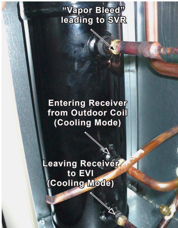
Figure 21: Receiver on Medium Cabinet (7.5T) Heat Pump (DPH)
