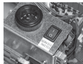
Service Switch in the OFF position
